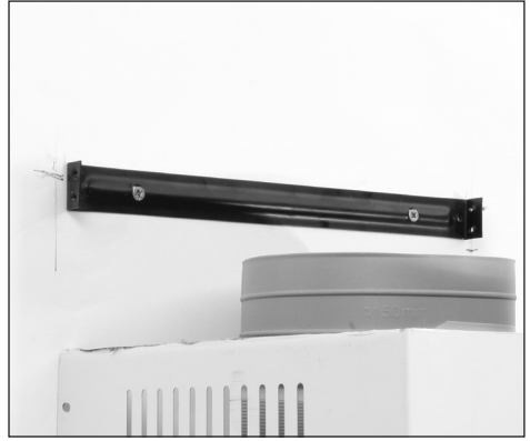
18. Centre top fixing bracket between surface lines, mark holes, drill & fix to wall
